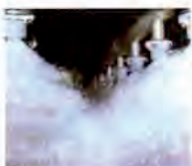
Tower desulfurization in power station
